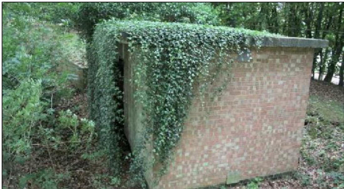
Figure 49: One of the magazines constructed within the grounds of The Frythe. These were constructed from Fletton bricks and roofed with reinforced concrete. 56
