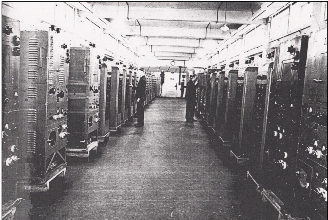
Figure 105: The interior of Station 53b transmitter at Godington. To ensure that equipment could be replaced quickly, the transmitters were mounted on platforms. 41
